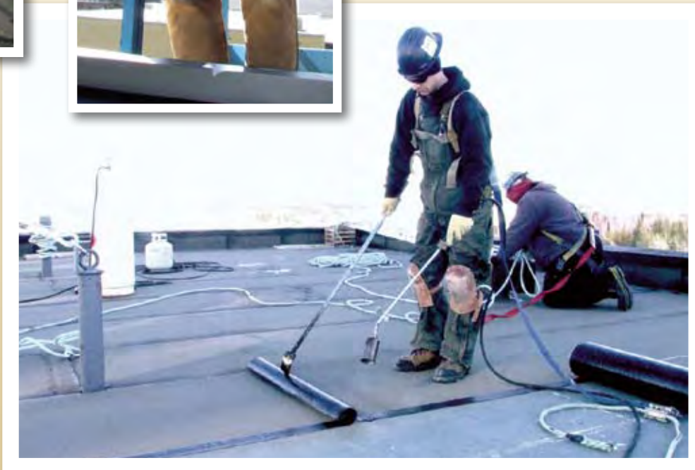
Tyler Comeau , a roofer with Unico Roofing Contractors, applies a vapour barrier on the roof of the Gallery Project site at 50 Avenue and 52 Street in downtown Yellowknife.
