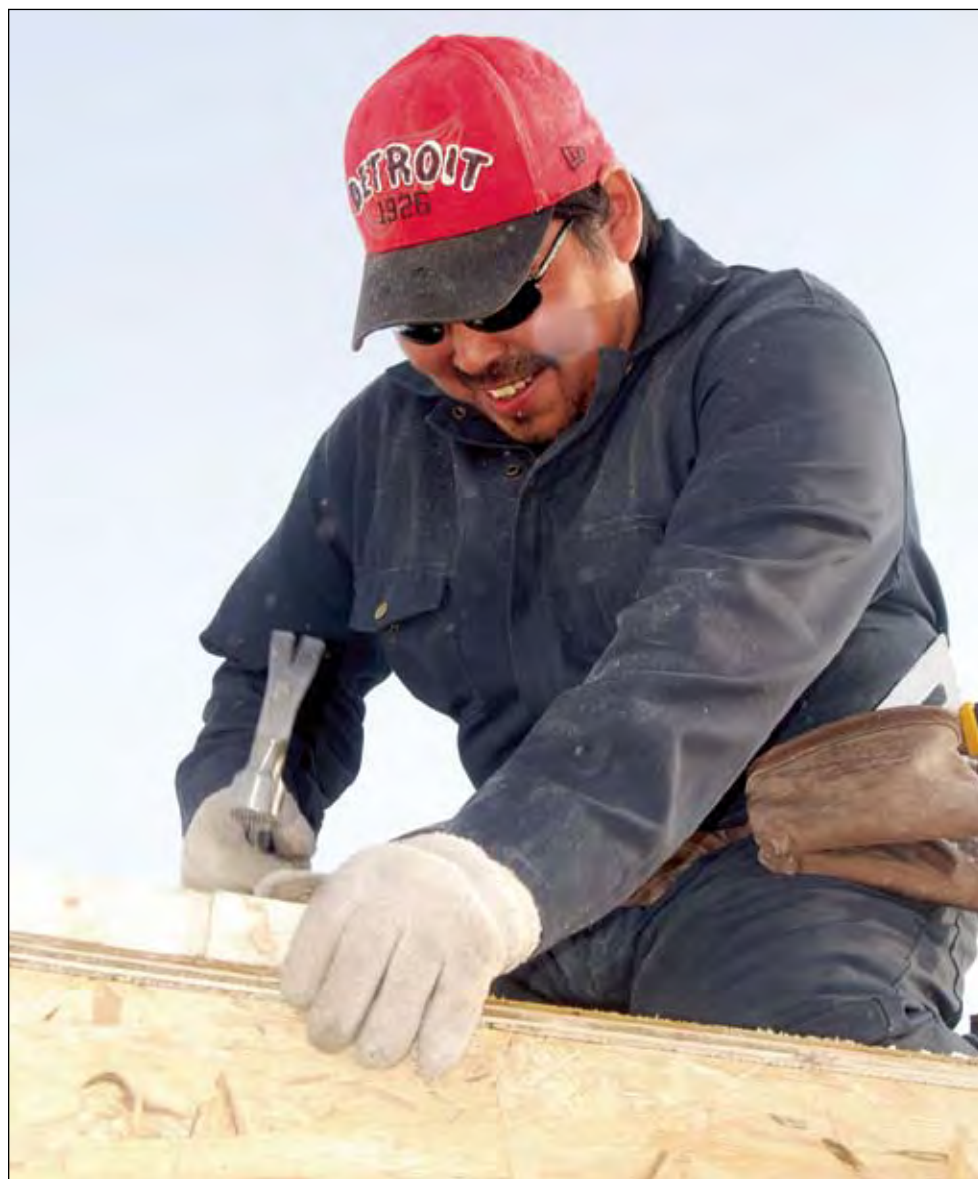
Nathaniel Mapsalak, a general labourer, hammers away at the construction site of a new apartment building in Repulse Bay. The building was erected by Naujat Co-operative Ltd. for the Nunavut Housing Corporation last summer.
